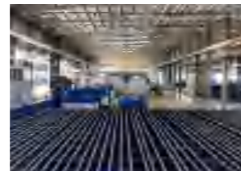
冷床 Cooling Bed
