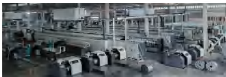
耐磨带焊丝生产设备 Welding wire for abrasive belt production equipment
